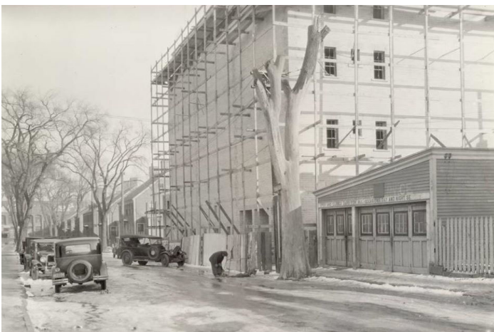
View of the rear of the Masonic Temple under construction along Worthen Street on December 14, 1928, looking toward the Merrimack Manufacturing Company millyard, the site of present-day River Place Towers. Merrimack Company boardinghouses, demolished in 1966, are visible on the right side of Worthen Street beyond the temple. (Photo – Lowell National Historical Park)
